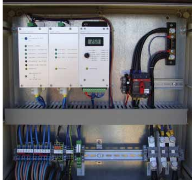
Example of a typical enclosure with 1 master control, 1 slave unit and 1 meter unit
