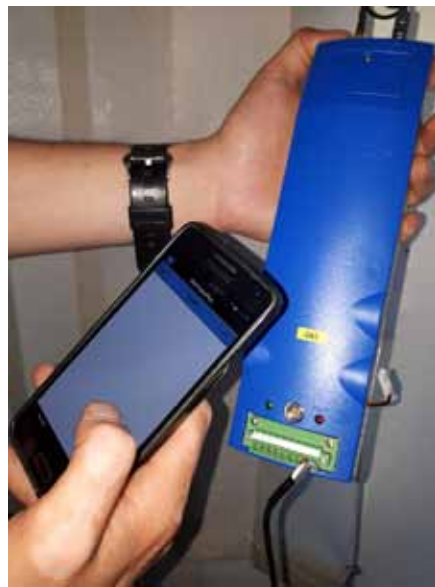
Controlling rectifier stations by mobile phone
